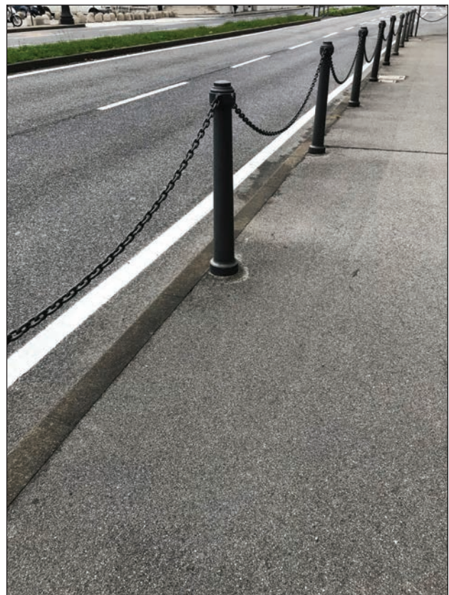
Figure 12: Urban furnishing (bollard chain) as barrier, when its presence cannot be checked by the white stick. Corso Cavour, Trieste, 2018 (Photo: G. A.).
