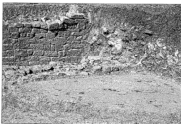
Sl. 11: Del tlaka in severni zid z ostanki ometa v prostoru 11.
